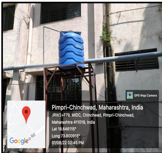
Water tank for drinking water daily
